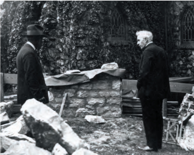
SELECTING STONE. Dr. Charles Robinson, rector, and Andrew Johnson, sexton, stand in the rubble after the demolition of the old parish house in the spring of 1925. They are examining rocks to be reused in the foundation of the new Christ Church.
